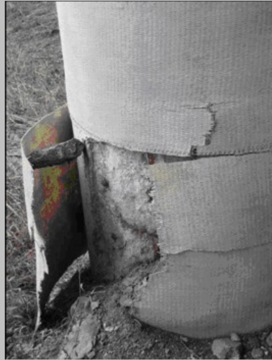
Fiberglass wraps provide support for deteriorating columns, but may not prevent further decay. WHRP will assess their net benefit.
